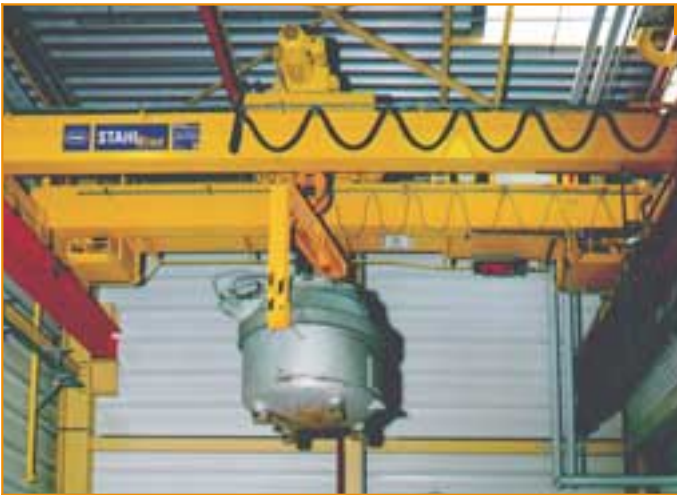
1 Foundry – Above-average demands: continuous operation, heat, dirt and loads up to 20,000 kg. The crane was equipped with a load display for even greater safety and productivity.
